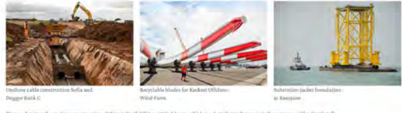
Photos showing the onshore construction of First Wind Offshore Wind Farm, which used similar techniques to those proposed for North Falls.
